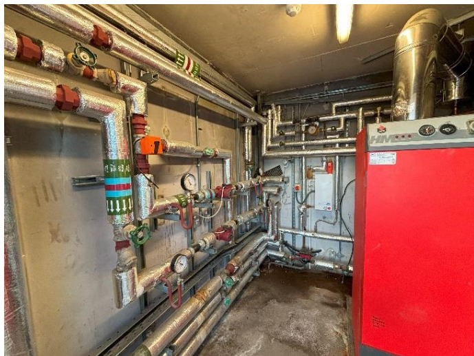
Figure 3-7: Ambulance Workshop boiler
