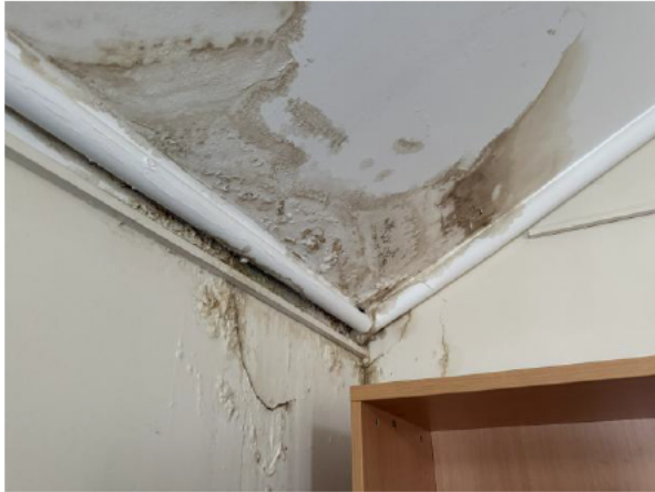
Photograph 11 – Water Ingress to First Floor
