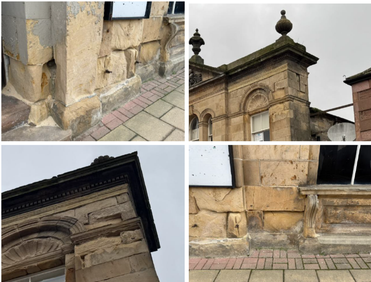
Photograph 04-07 – Stone Weathering to Front Elevation
