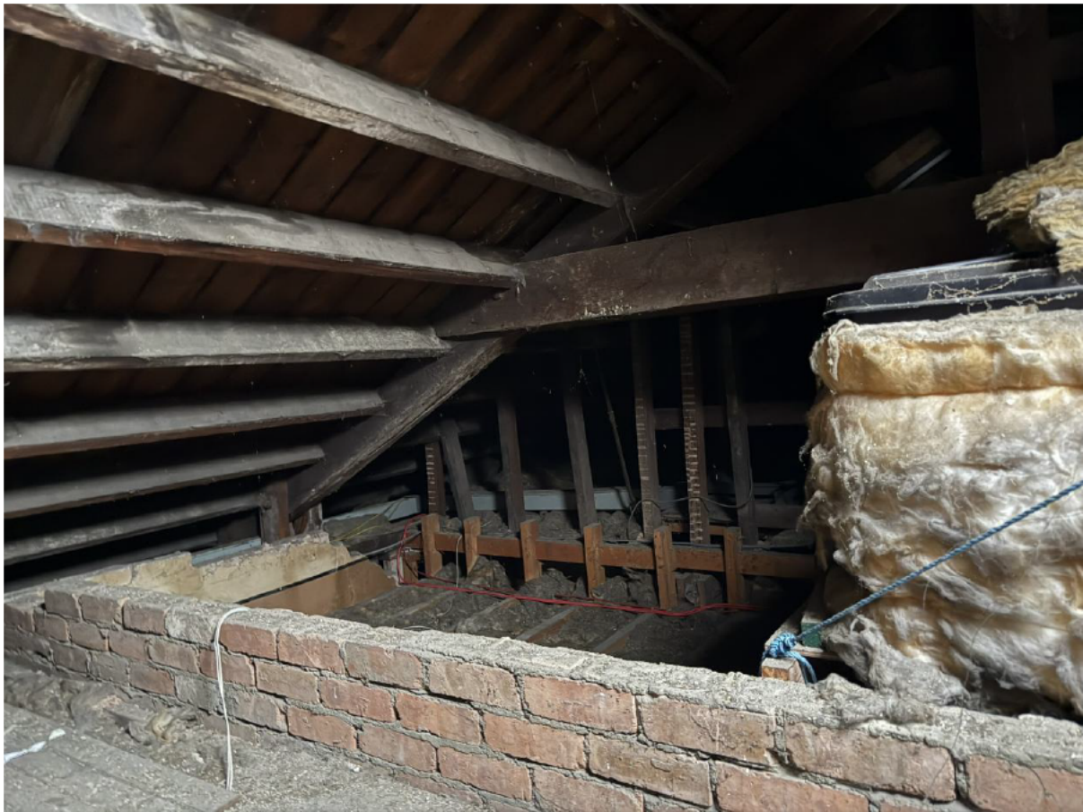
Photograph 13 – Evidence of Water staining to King Post Truss and Purlins
