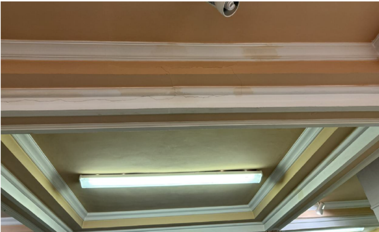
Photograph 10 – Hairline Cracking to First Floor Ceiling
