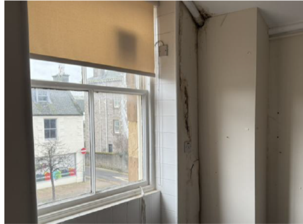
Photograph 12 – Water Ingress at Front Corner
