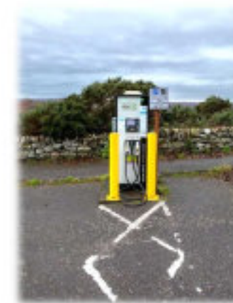
Electric Vehicle Charging Point at Tongue Hotel
